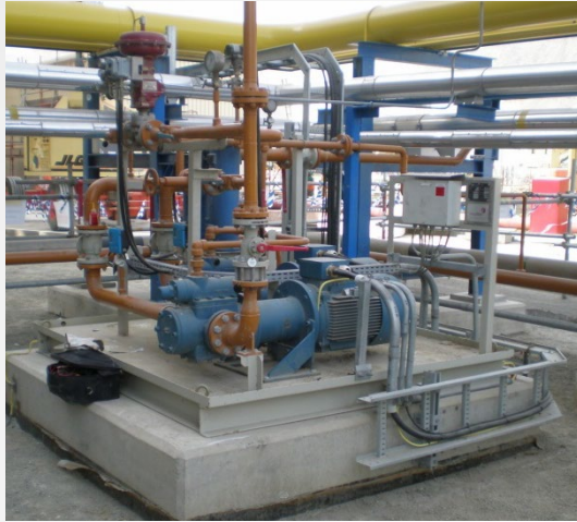
High Pressure Pumping Set
