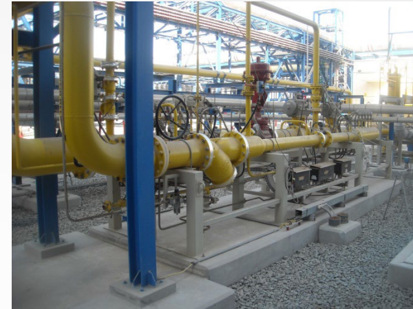
Flow control and shut off valve train
