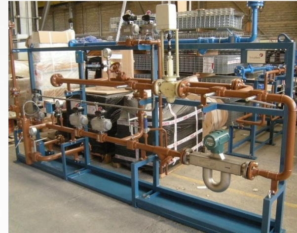
Flow control and shut off valve train
