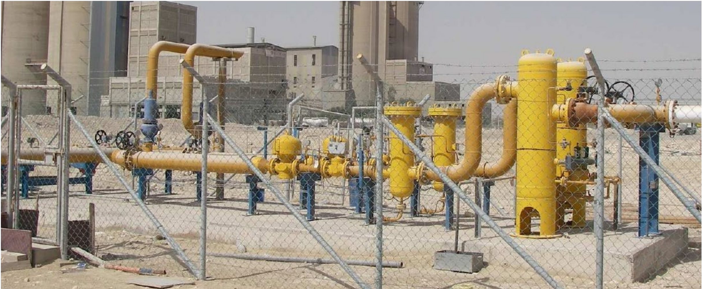
GAS PRESSURE REDUCING STATION
