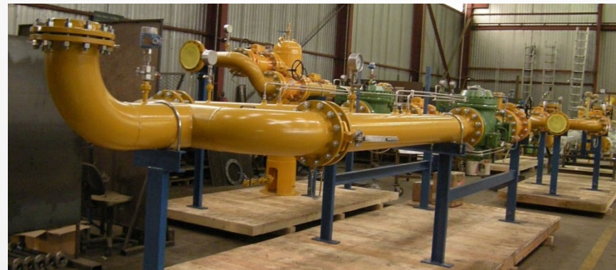
Pressure Reducing Station
